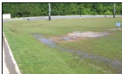
Poor field drainage on a soccer field improperly constructed. Photo: Tony L. Strickland, CSFM
